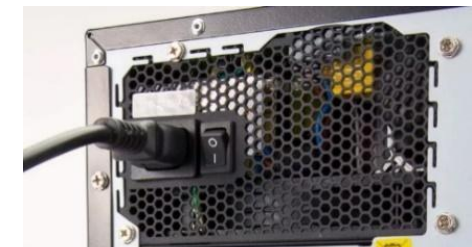
Figure 9: Power Supply in the ON position
